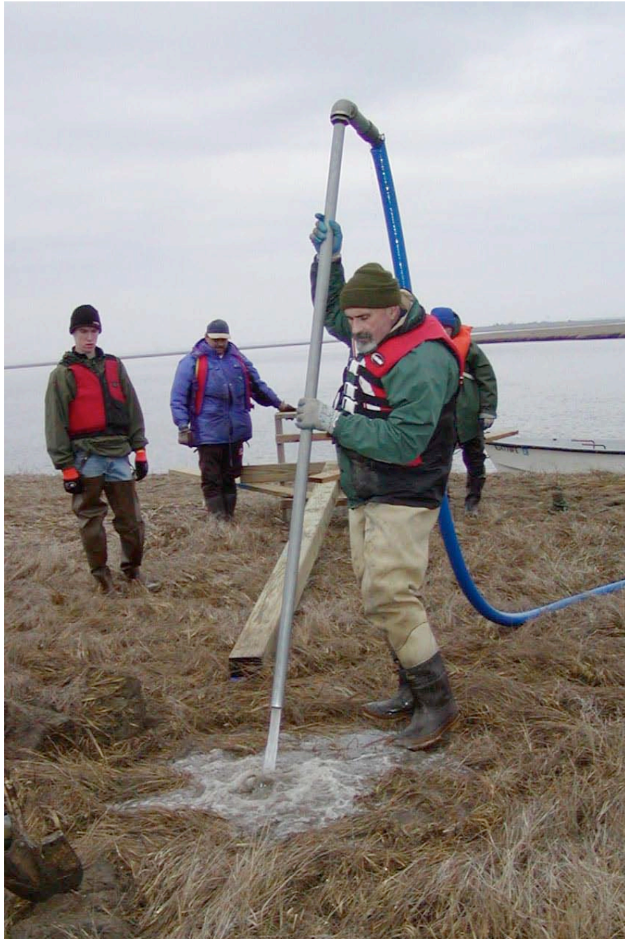
Attached to the pump's hose is a 6' galvanized "L" shaped pipe. One individual will allow the water to do the work.
